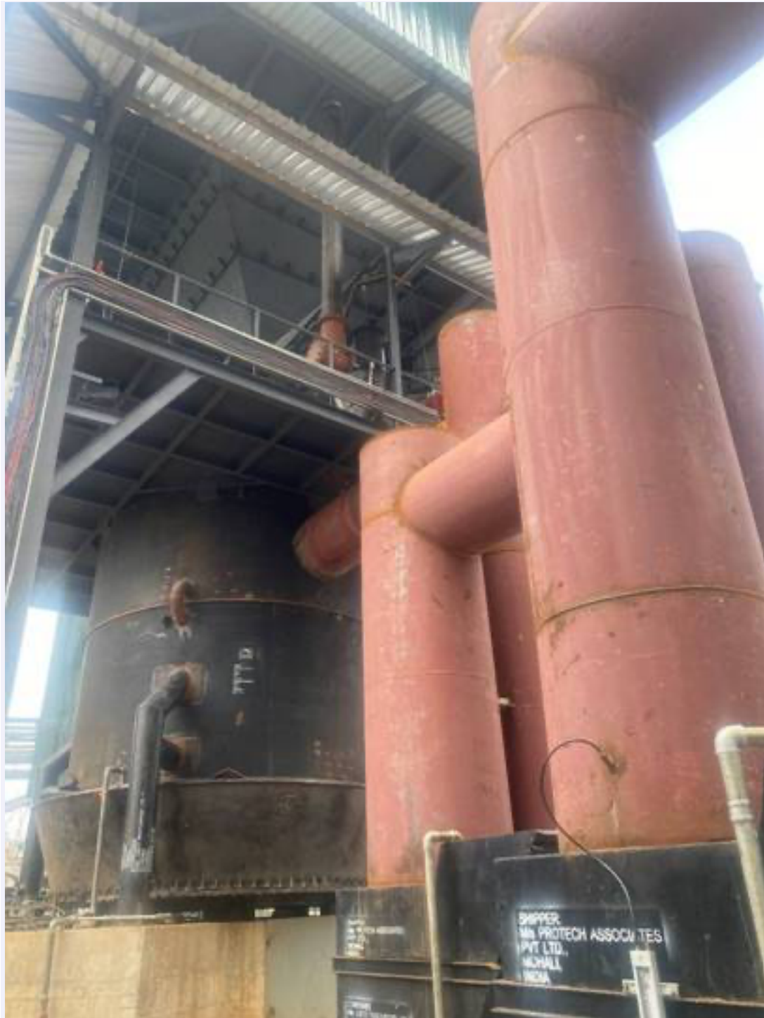
Figure 3: View of gasifier and gas ducting connecting gasifier to lime plant.
