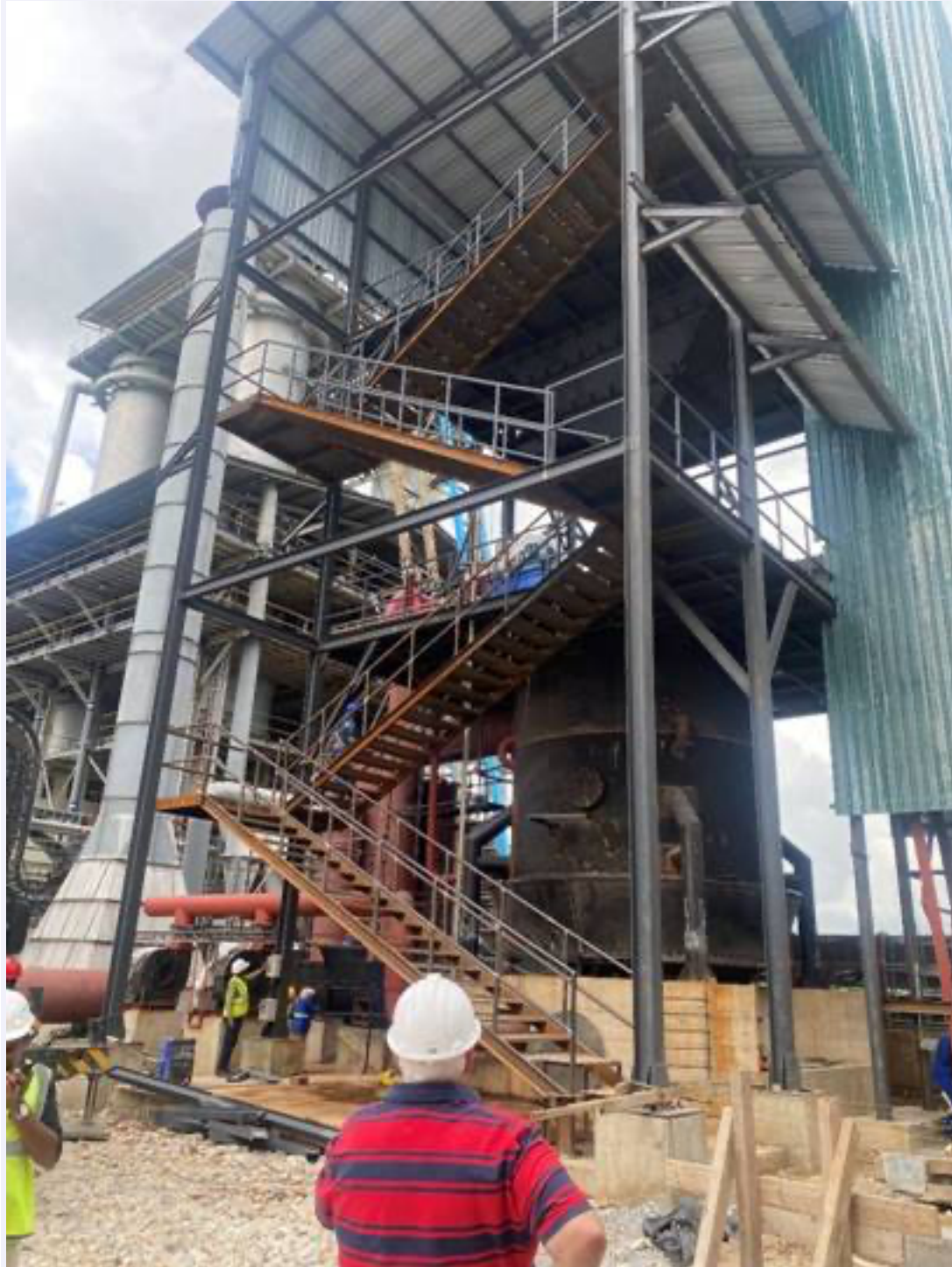
Figure 5: View of gasifier with lime plant in the background.
