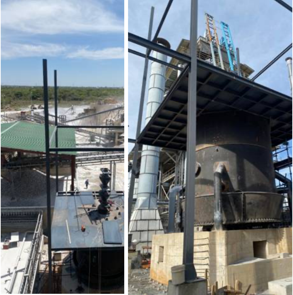
Figure 3: View of the steel structure and 1 st platform from the lime plant (left); view of the gasifier with 1 st platform (right).
