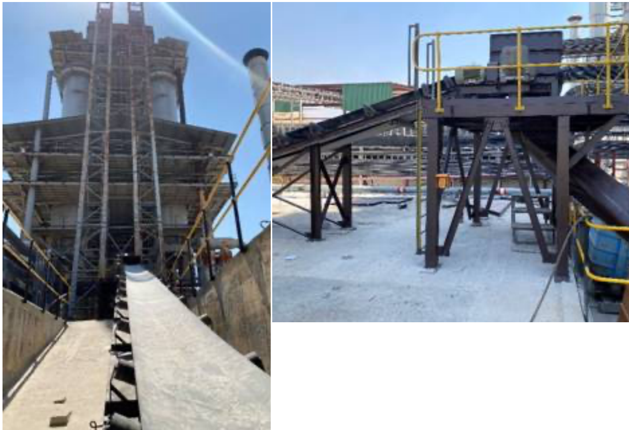
Figure 1: View of newly installed conveyor belt (left) and feeding arrangement into skip hoist (right). Two new brakes for the skip hoist motor arrived on-site in early August 2024 and have since been installed (Figure 2), replacing the original single brake. Brake testwork is planned for September 2024.
