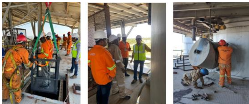
Figure 3: Protech inspecting the kilns and stripping the burner ports to be modified for coal gasification (Source: Limeco, 2024).
